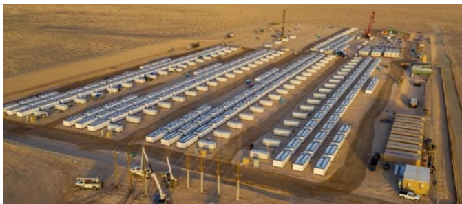
Figure 3: Crimson Storage, a BESS facility in Riverside County, California
